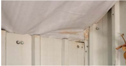
Fig. 14 Sharp edges in cladding [15]
