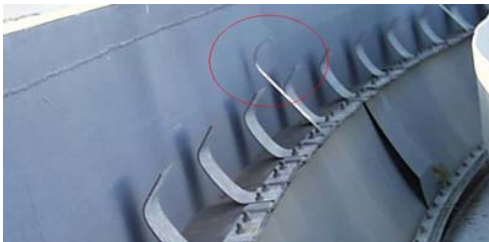
Fig. 2 Shunt not making contact with Out-of-Round Tank Shell [1]
