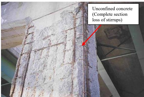
Fig. 2 Effect of corrosion on reinforced concrete column [5]
