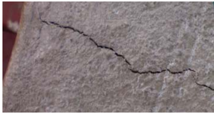
Fig. 8 Example of plastic shrinkage cracking
