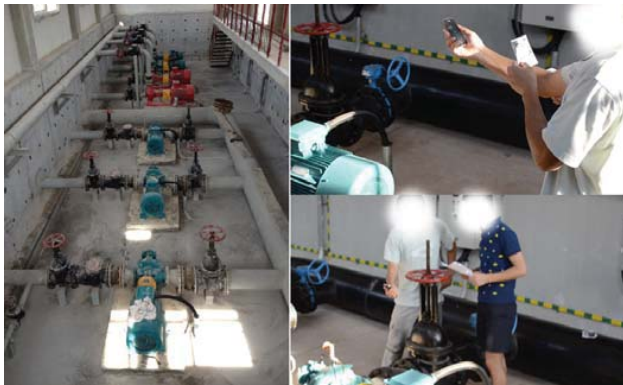
Fig. 5 Integrated pump house and pump test
