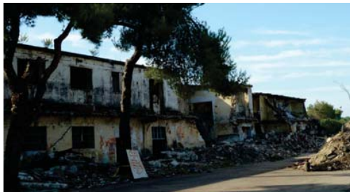
Fig. 11 Ex-American collapsed hospital, Calambrone, Italy
