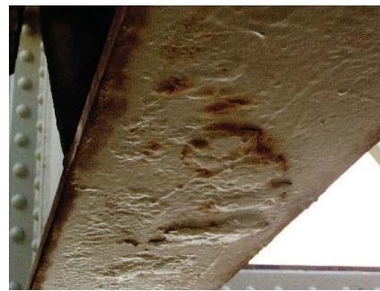
Fig. 1 Appearance of Under-film Corrosion
