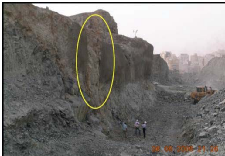
Fig. 2 View of the site condition of the site, the yellow circle indication the failure section
