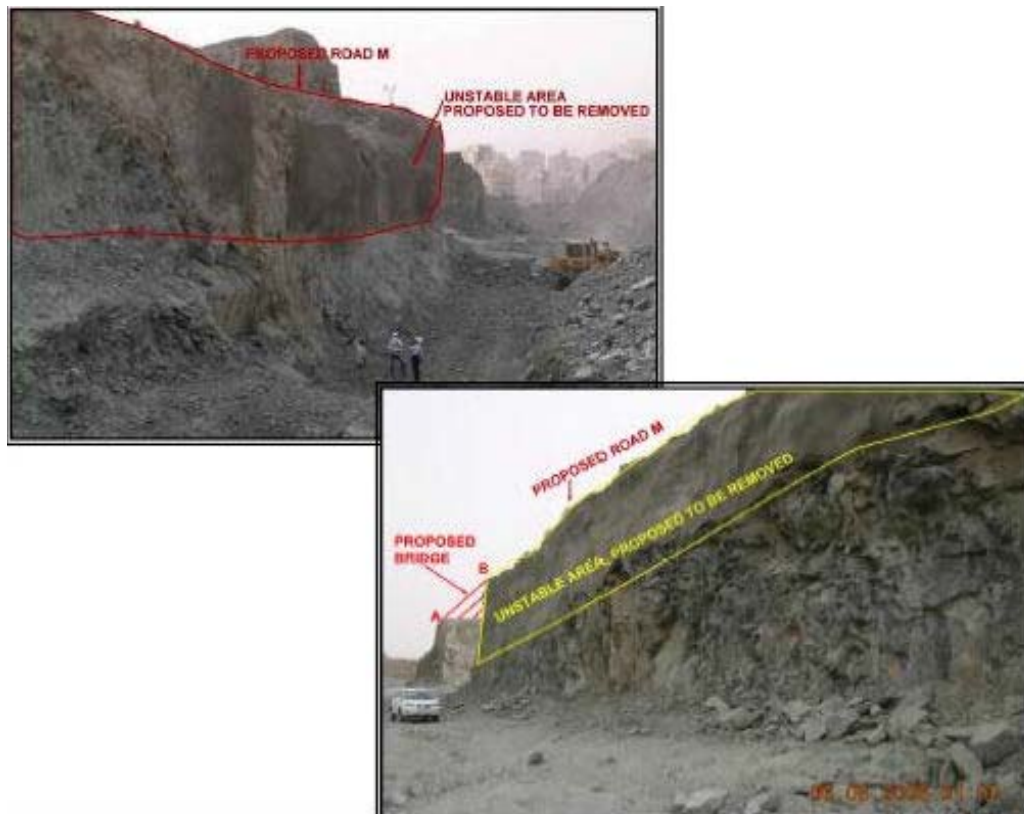
Fig. 8 The proposed mitigation measures for the unstable slope along the site - the concrete-covered upper part of the slope to be removed, supported with MSE wall and backfill with suitable fill materials
