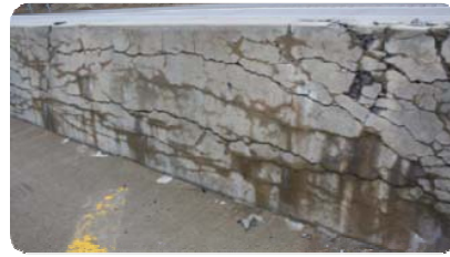
Fig. 5 Deterioration in Arkansas Highway Projects
