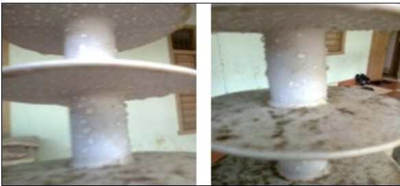
Fig. 4 Appearance of water droplets on the surface of insulator in the early morning hours
