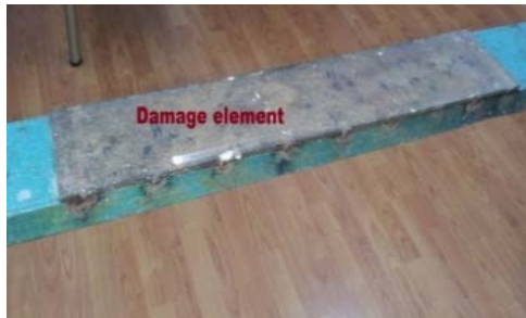
Fig. 4 Damage element in beam
