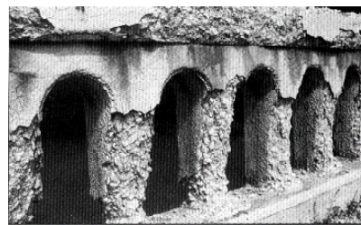
Fig. 1 Typical example of concrete deteriorated from freeze-thaw actions. (Non-air-entrained concrete railing, PCA vol. 19/1 1998)
