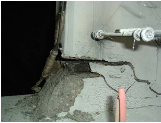
Fig. 3 Fallen state of the parts of the concrete at the upper corner of the corbel of the DP1R specimen
