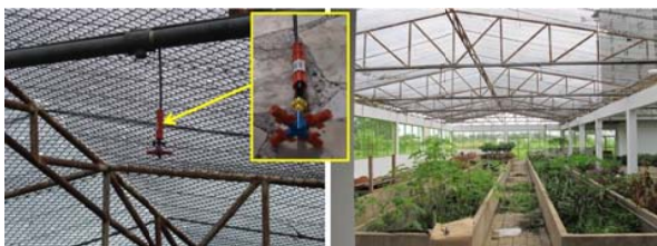
Fig. 5 The Fogger Installed Inside the Greenhouse
