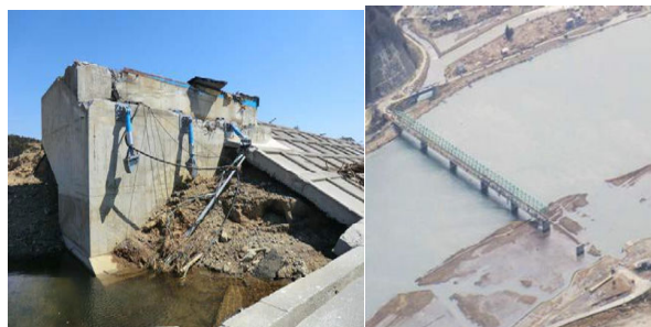
Fig. 2 Washed away girder bridge and truss bridge
