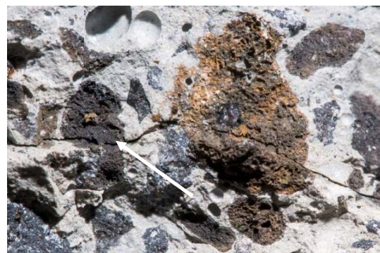
Fig. 5 State after testing – crack in cement past and lightweight aggregate
