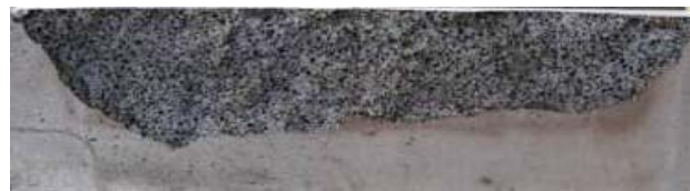
Fig. 4 State after testing – spalled concrete
