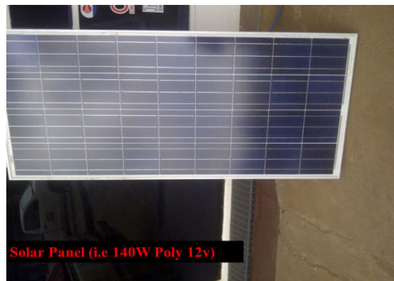
Fig. 6 Solar (PV) array component of the groundwater pump
