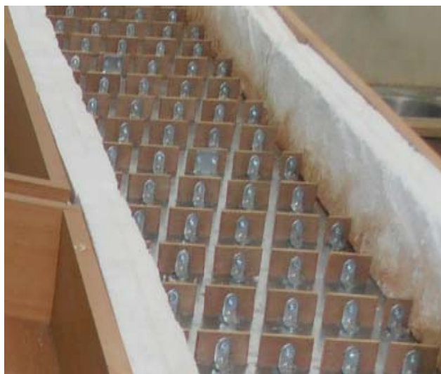
Fig. 3 Photograph of installed baffles (Taken from downstream perspective)
