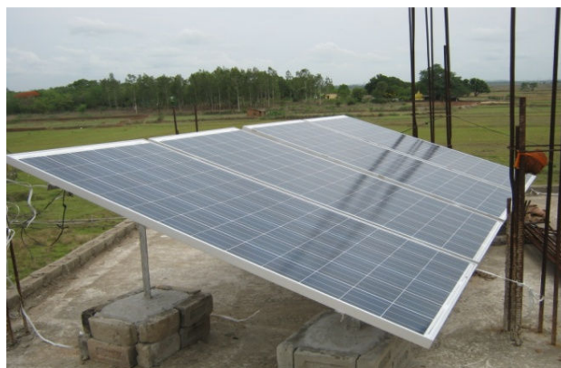
Fig. 8 Rooftop PV system
