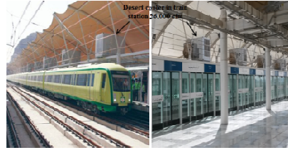
Fig. 6 Evaporative cooling units in the train station
