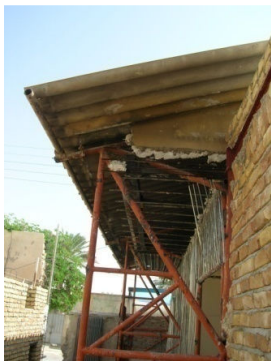
Fig. 19 Difficulties in attaching new parts to the employed alien roof system in original PEHs
