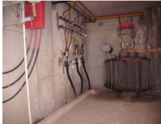
Fig. 2 Magnetic field measurement at distribution substation
