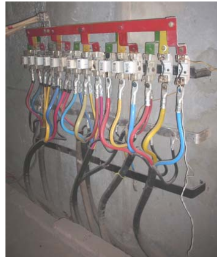
Fig. 3 Low voltage panel view
