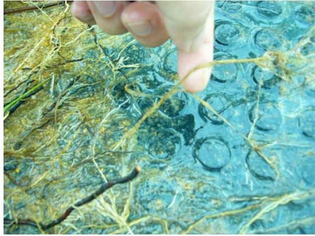
Fig. 7 Roots which seemed to have anchored on the membrane
