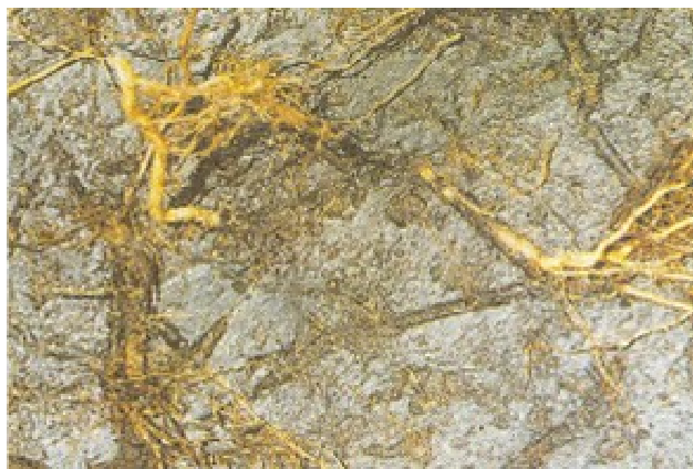
Fig. 1 Roots leaving impression on waterproofing membrane, adapted [10]
