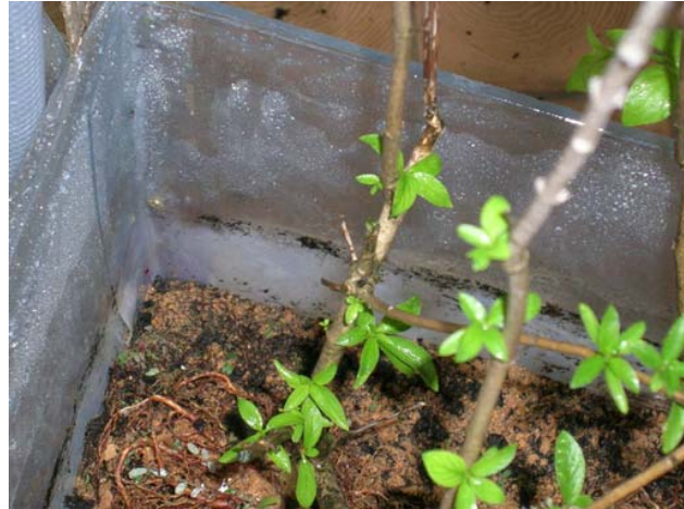
Fig. 11 Growth observed between joints of the membranes
