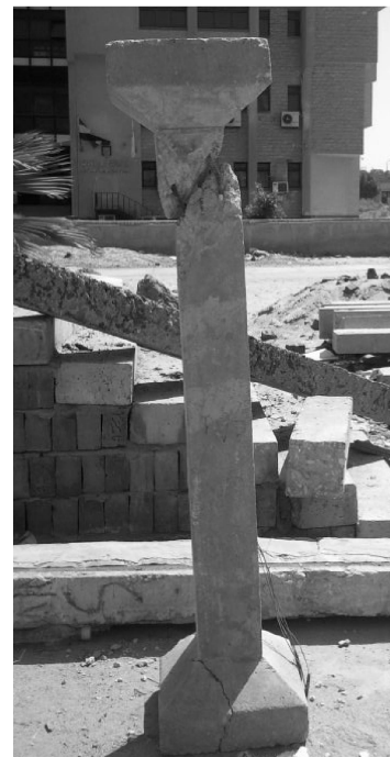
Fig. 18 Failure mode of axially loaded column
