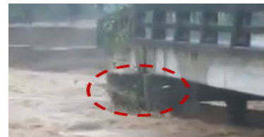
Fig. 19 Case 3: the bridge failure in flood
