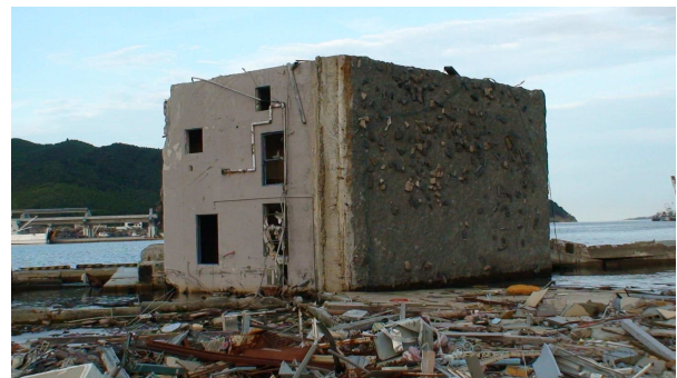
Fig. 22 Detail of slab foundation of collapsed building
