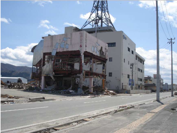
Fig. 13 Destruction of wall panels
