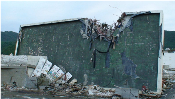
Fig. 24 Detail of impact on the building
