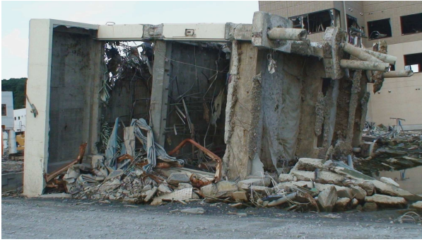
Fig. 23 Collapse of 2 story RC building
