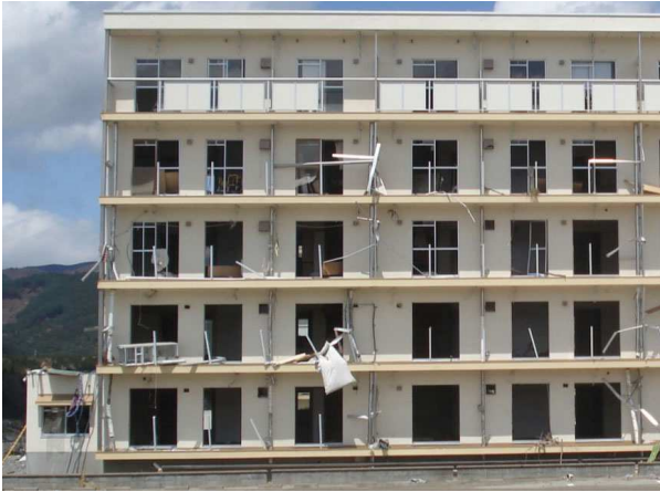
Fig. 18 Detail of damages on balconies
