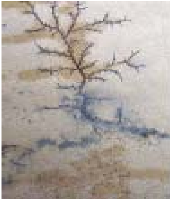
Fig. 3 Case of tracking discharge in wet insulation
