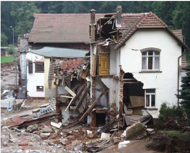
Fig. 2. Example of a close to collapse building with intact floor parts. Photo: Michael Markus.
