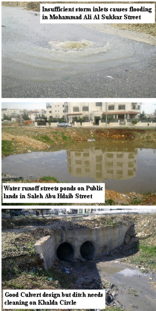
Fig. 4 Example Problems of the roadway drainage systems in Site 2
