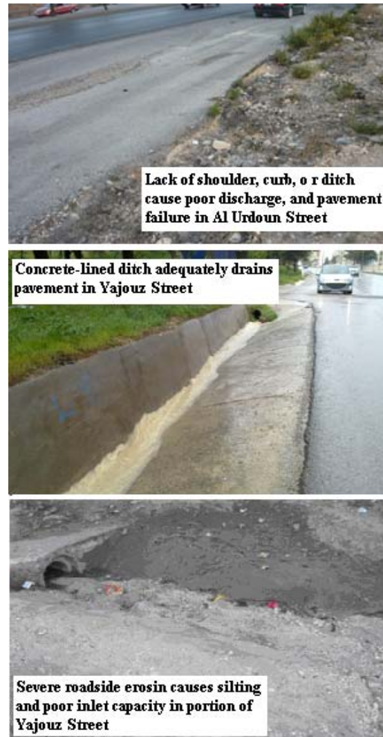
Fig. 5 Example Problems of the roadway drainage systems in Site 3
