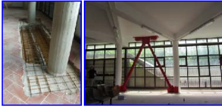
Fig. 17 Construction of the additional R/C beam in one of the two DB alignments parallel to x in the pilotis wing
