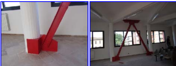
Fig. 18 Detail and general views of the other DB alignment parallel to x in the pilotis wing
