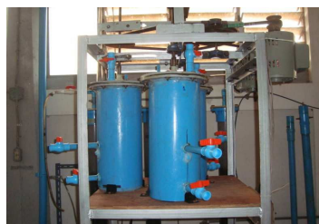
Fig. 2 the anaerobic reactors
