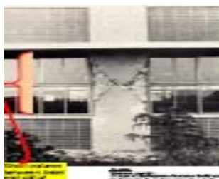
Fig.4. large window openings AND SHORT COLUMN
