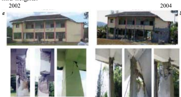
Fig. 10.a.Severe Cracking and Damage to soft first storey columns of Nabagram Panchayat Bhavan building primarily due to 'missing' ties in 2002 earthquake, b.more damage in 2004 earthquake to same columns which were 'retrofitted'[9].
