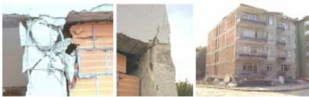
Fig. 9.Observed effects of interaction between infills and bare frame a)shear failure of column , b)exterior joint shear damage(Bonefro,Molise,2002) , c)global collapse for soft storey mechanism(Izmit,1999).
