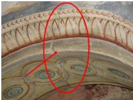
Fig. 16 Cracks at arches
