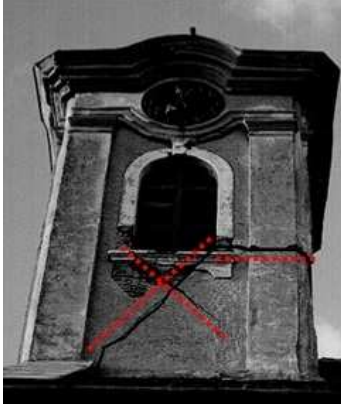
Fig. 15 Cracks at bell tower
