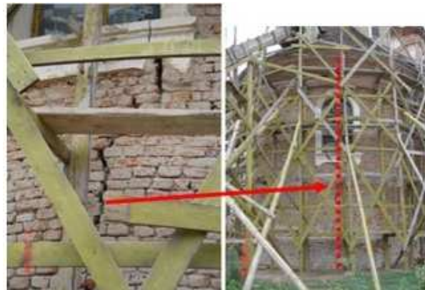
Fig. 14 Cracks at the eastern wall
