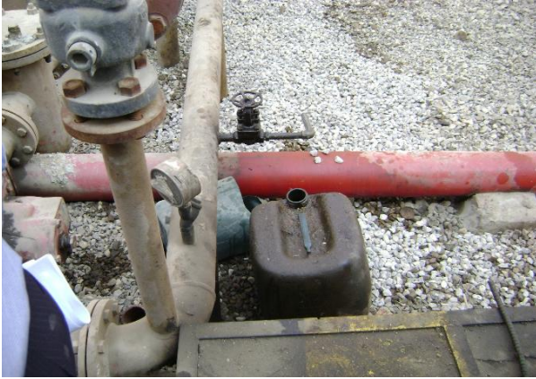
Fig. 10 Housekeeping of tank zone was found poor
