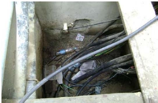
Fig. 14 Electric cable trench was found uncovered
