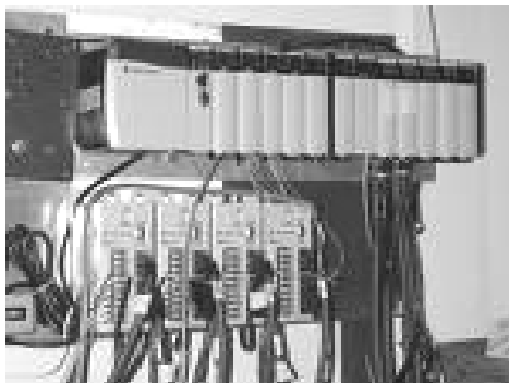
Fig. 2 A large PLC
