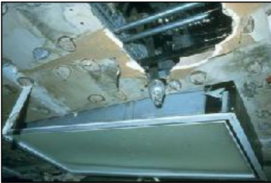
Fig. 2 Piping Failures in 1994 Northridge Earthquake (Miranda, 2004)
