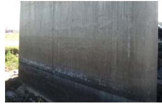
Fig. 7 Transverse cracks Pier #11
