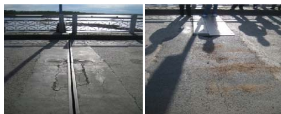
Fig. 11 Serious damaged bridge deck expansion joint
