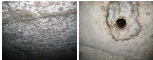
Fig. 9 (a) the internal box water drainage damage
