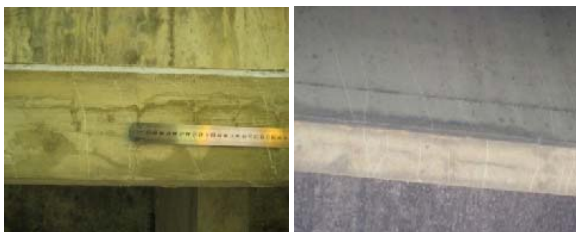
Fig. 9 (c) T beam cross-cracks in the region
