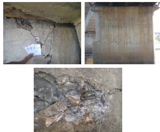
Fig. 4 Damage of concrete bridge abutment #14 and pier No. 5
