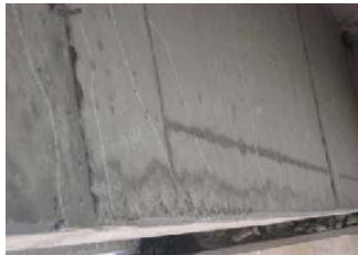
Fig. 9 (b) T beam cross-cracks in the region
