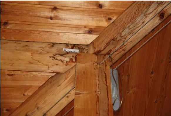
Fig. 1 Convective moisture ingress through a leakage at the connection point of bay and timber frame
