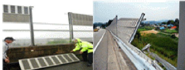
Fig. 1 Failure of soundproof wall
