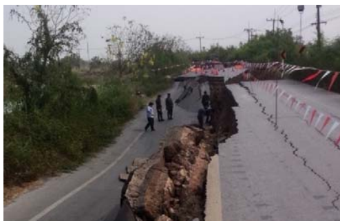
Fig. 1 Road along the canal no.13 collapsed
