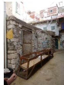
Fig. 4 Ruins of Sayied Darwish historic building
