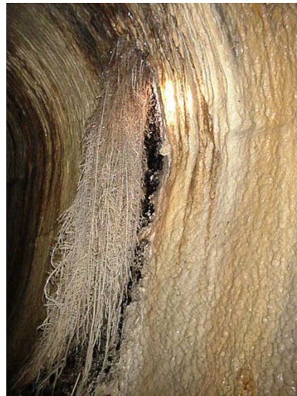
Fig. 12 Obstruction and fissuration of the canalisation by vegetation (weak maintenance).
