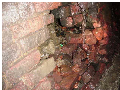
Fig. 13 Destruction of the wall of culvert by the water pressure (Absence of pore drainage in the wall: weak maintenance).
