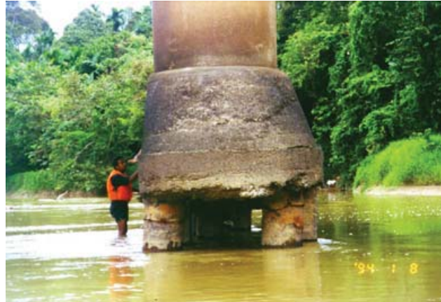
Fig. 4 General scouring of river bed at Sg. Jeniang, Kedah
