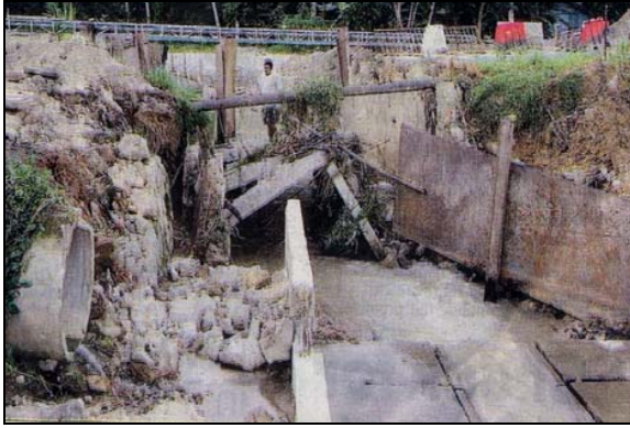
Fig. 6 Bridge in Seremban, Negeri Sembilan collapsed due to heavy rain and flooding [20]
