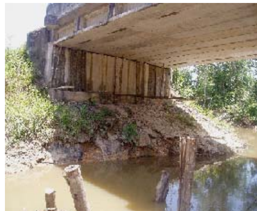
Fig. 5 Bridge failure due to scouring at Bokah Rasau Stungkor Road, Kuching, Sarawak [20]
