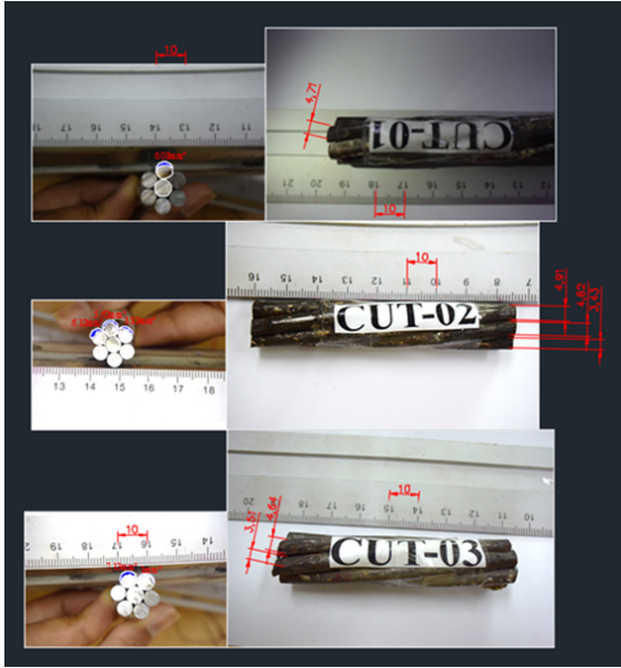
Fig. 3 Evaluation of corroded section
