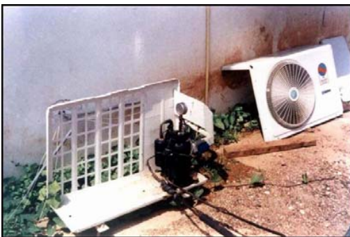
Fig. 3 Photograph of condensing unit of M-AC
