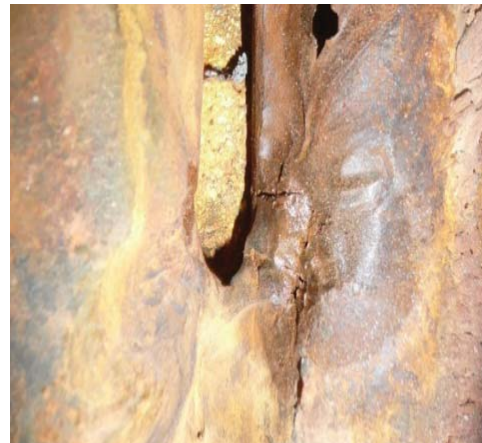
Fig. 1 Cracks at fin tip of tubes membrane
