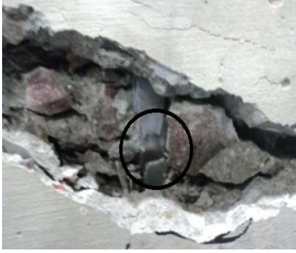
Fig. 5 the necking phenomenon of steel strips
