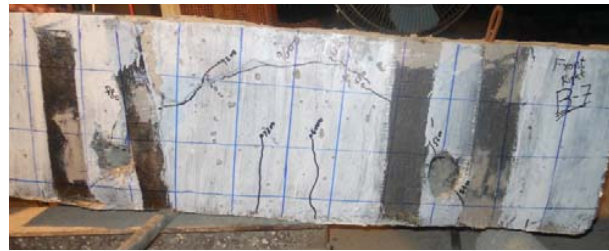
Fig. 11 Crack pattern of beams with opening below NA
