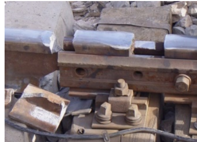
Fig. 1 Crack in rail bolt hole
