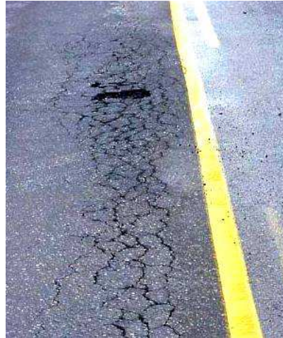
Fig. 4 fatigue causes pothole
